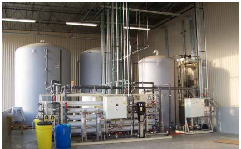
Reverse Osmosis System
