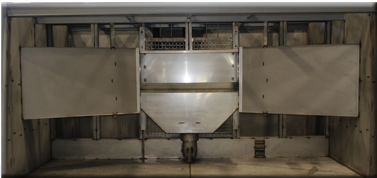
Fixed AutoWeir installed in paint recirculation tank
