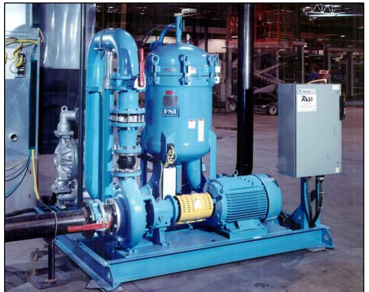
Stand-Alone Pump Skid & Filter
